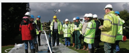
CMT Installation and training as part of a “Multilevel Course” given by the University of Cranfield at Silsoe, U.K., in conjunction with Waterra (UK), British Geological Survey & Norwest Holst.
